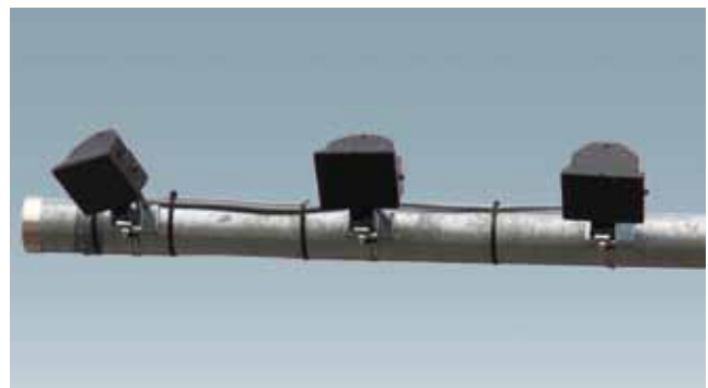
Road traffic detectors cover the danger zone
