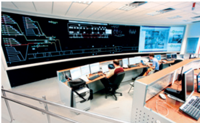
Siemens technology: ViaQuatro control room in São Paulo.
