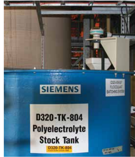
SITRANS Probe LU ultrasonic transmitter tracks the level of flocculant chemical.
